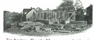
Two days later—November 5th—two men on the job ready to start sheathing
